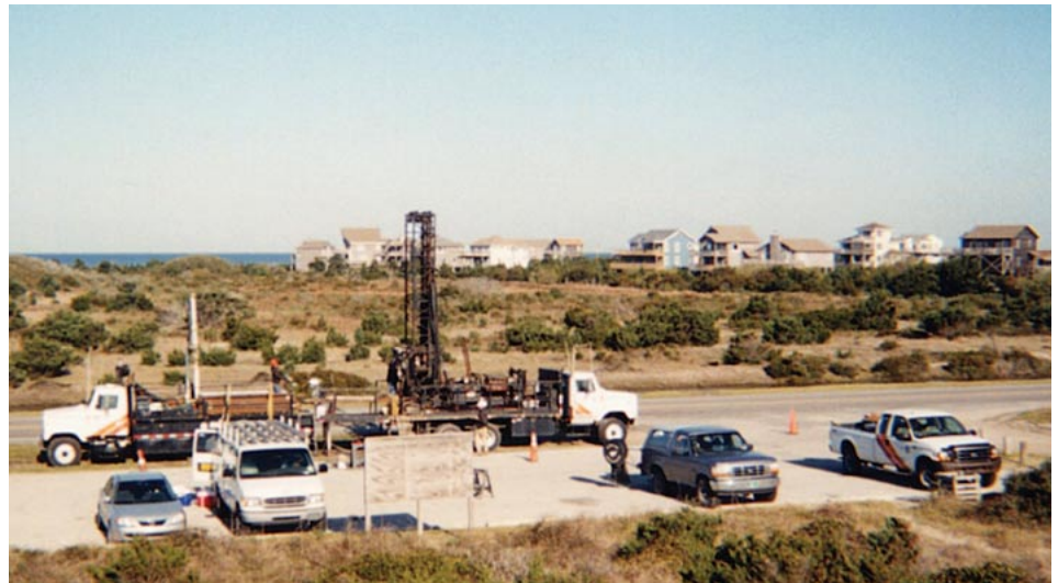
Roto sonic-drilling rig set up adjacent to dunes south of Avon, NC.
