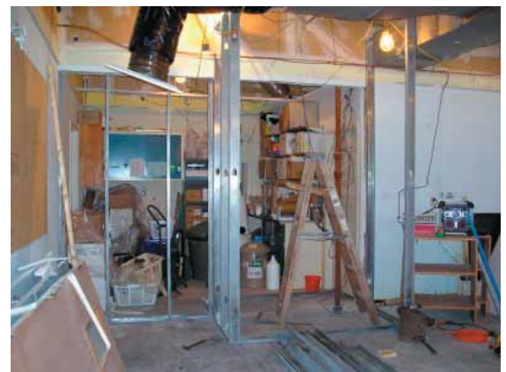
A view of the larger clean room undergoing renovation. The facility will have two rooms, the larger at Class 100,000 and the smaller at Class 10,000. The total area of the facility will be 500 ft 2 . Photograph by Sarah Kelsey .
