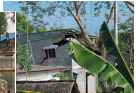
▲ Earthquake damage in Banda Aceh, such as this cracked wall, was much less severe than tsunami damage. (January 21, 2005)
