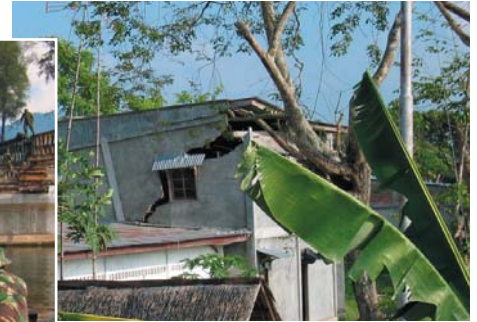
▲ Earthquake damage in Banda Aceh, such as this cracked wall, was much less severe than tsunami damage. (January 21, 2005)
