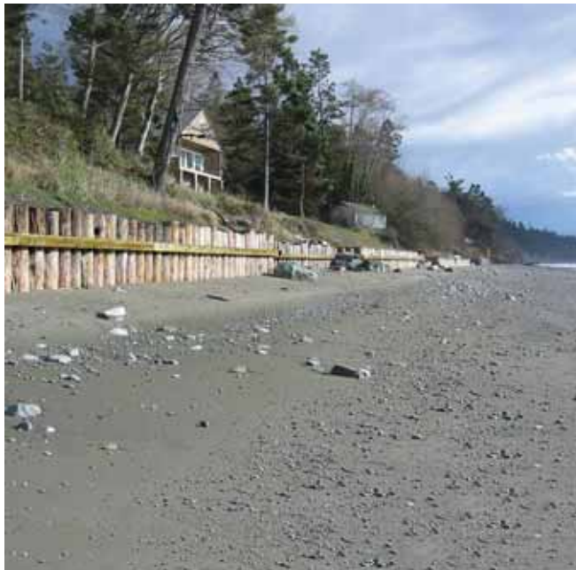
Photograph from the cover of the new USGS report shows timber-pile bulkheads built to protect residential property from erosion at Ledgewood Beach, west side of Whidbey Island, Puget Sound. Photograph by Hugh Shipman , Washington Department of Ecology.
