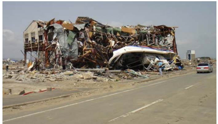
Building damaged by the tsunami in Yuriage. The tsunami flow depth here was approximately 8 m (26 ft).
